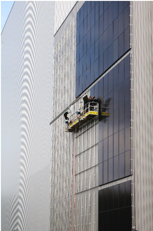
Photo 3: Photovoltaic system_south facade.jpg
